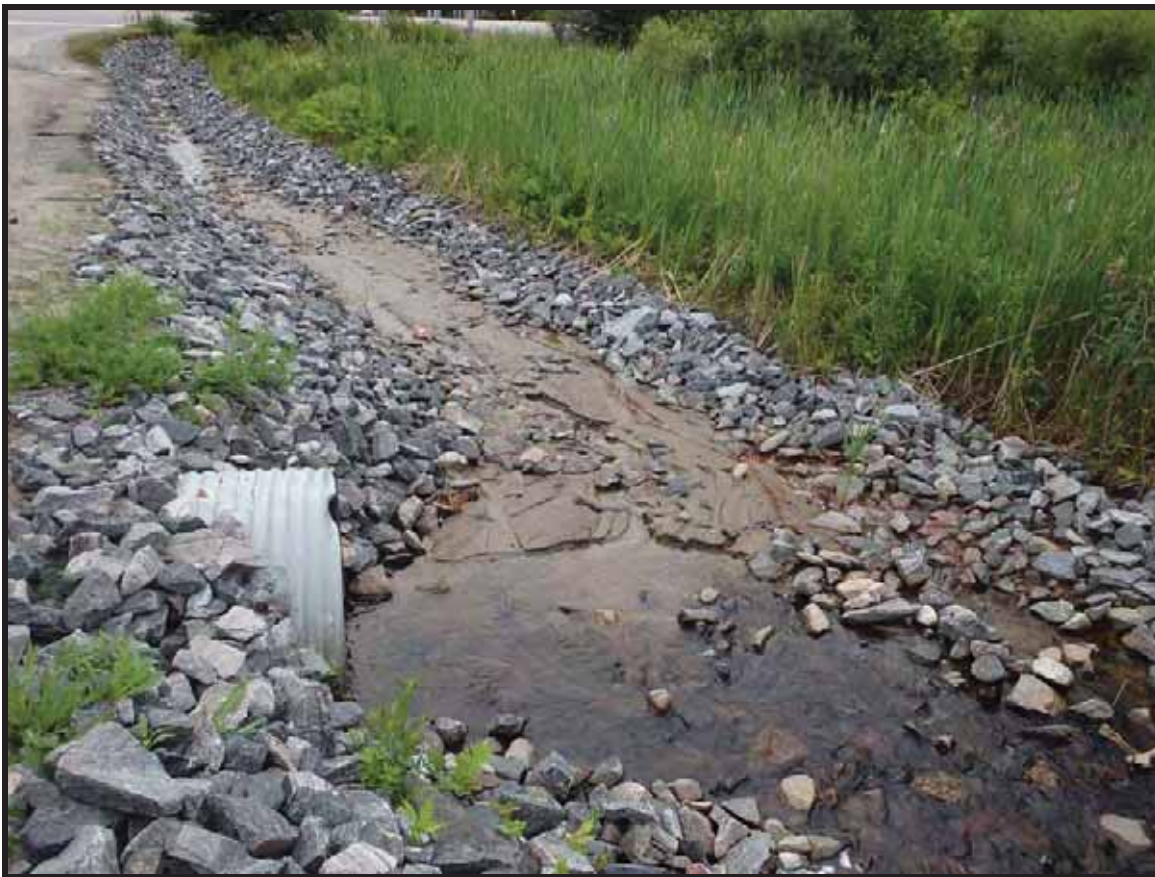
Photograph 1 Sediment movement into Chippewa Creek upstream of Marsh Drive
